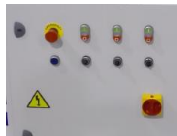
PANEL DE CONTROL/ CONTROL MACHINE
