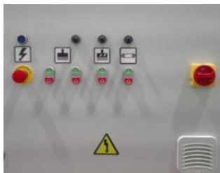
CONTROL MÁQUINA MACHINE CONTROL
