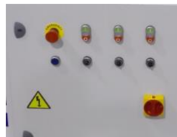
PANEL DE CONTROL/ CONTROL MACHINE
